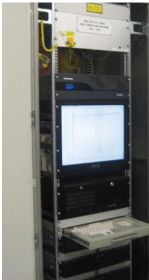
Fiber-optic control panel
