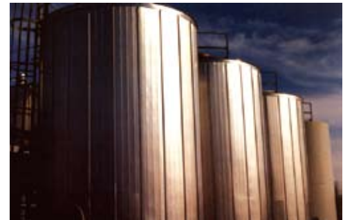
Vertical Lock-Seam Tank Insulation
